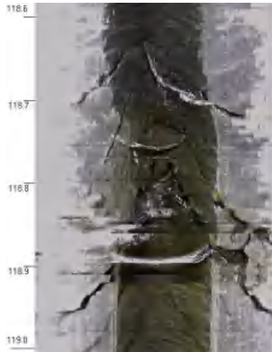
图8.3-17 118.64~118.98/97.2m深处垂向裂隙
